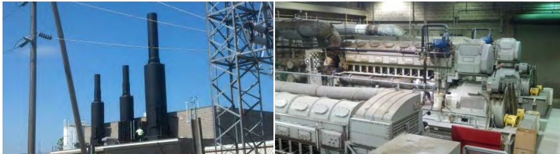
Falling Spring Generation Station - Unit #7 (1999) in Foreground, #6 (1968), and #5 (1968)
