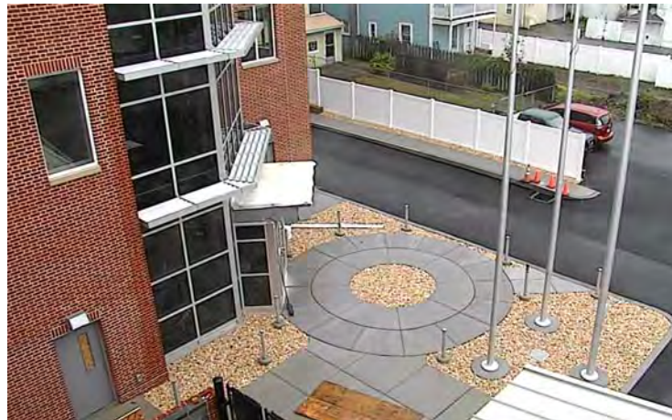
Newly completed rear parking lot entrance & plaza for the Utility Departments' Addition for City Hall
