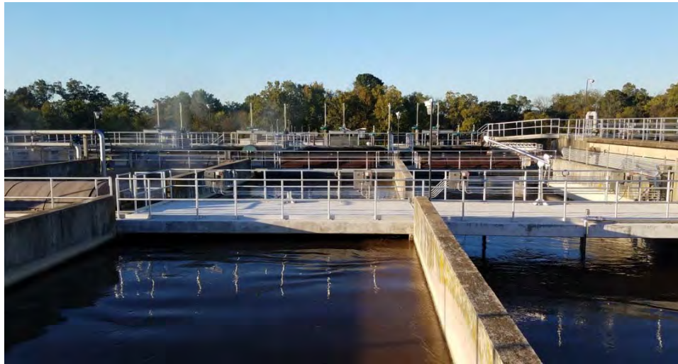
Modified VLR Tanks in Operation in 2017
