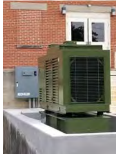
Back-up Generator at Recreation Center
