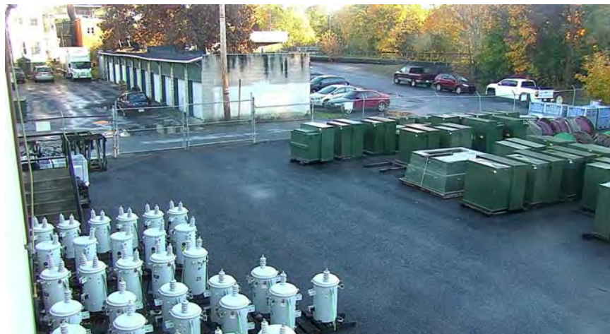
Electric Department Transformers and Cable Stored Securely at Warehouse
