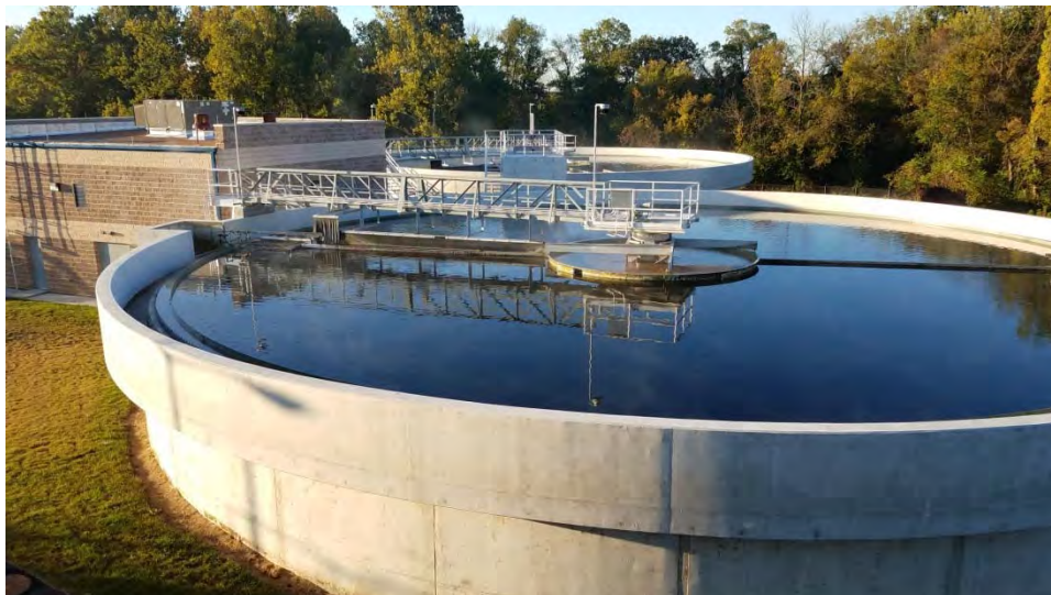
New Clarifies in Operation in 2017
