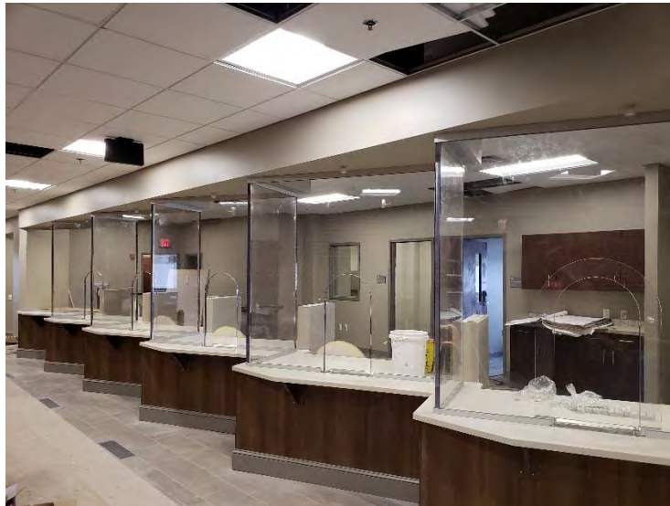
New teller stations under construction in the Utility Departments' Addition to City Hall
