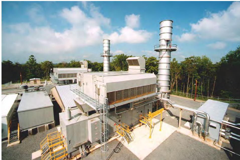
Orchard Park Generating Station (OPGS)
