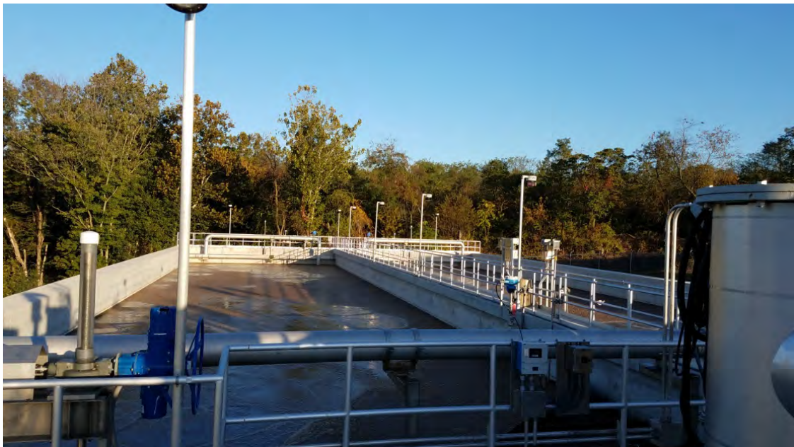
Post Aeration Tank in Operation in 2017
