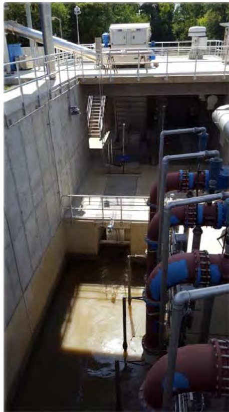
New Headworks in Operation Beginning in 2016
