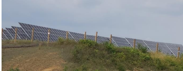
Chambersburg Solar Center – Photovoltaic Panels
