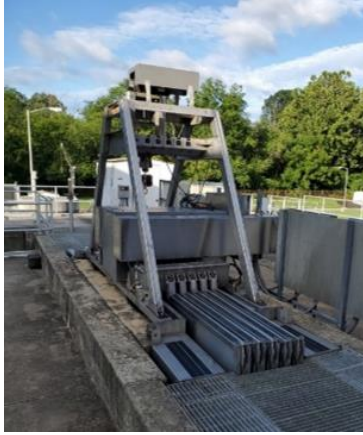
Aging Equipment – UV Disinfection
