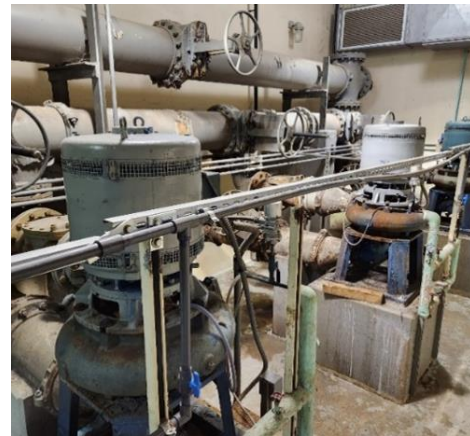
Aging Equipment – Old Headworks
