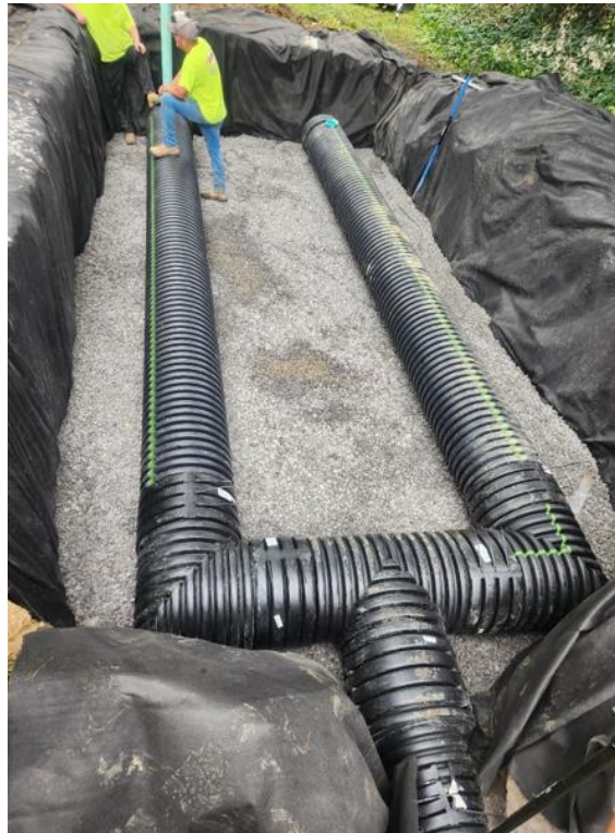
Water Street Infiltration Bed
