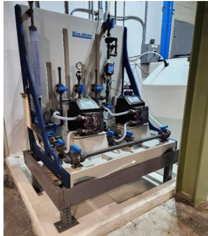
New Chemical Feed Equipment Installed in 2023
