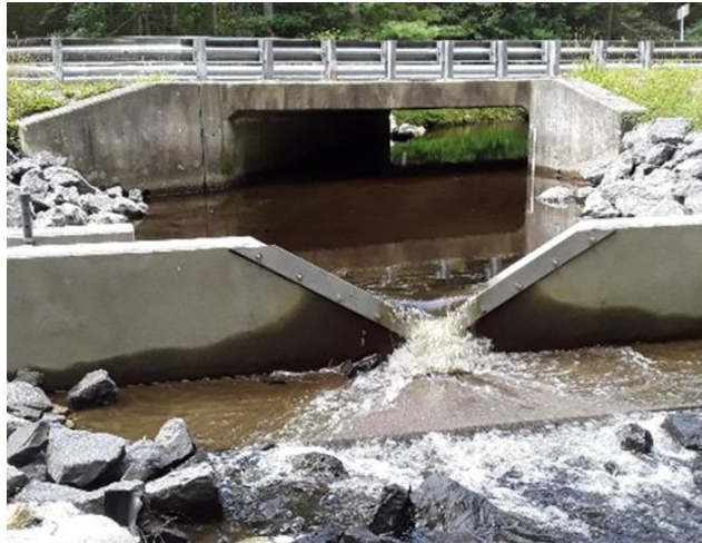
Conococheague Weir in Operation
