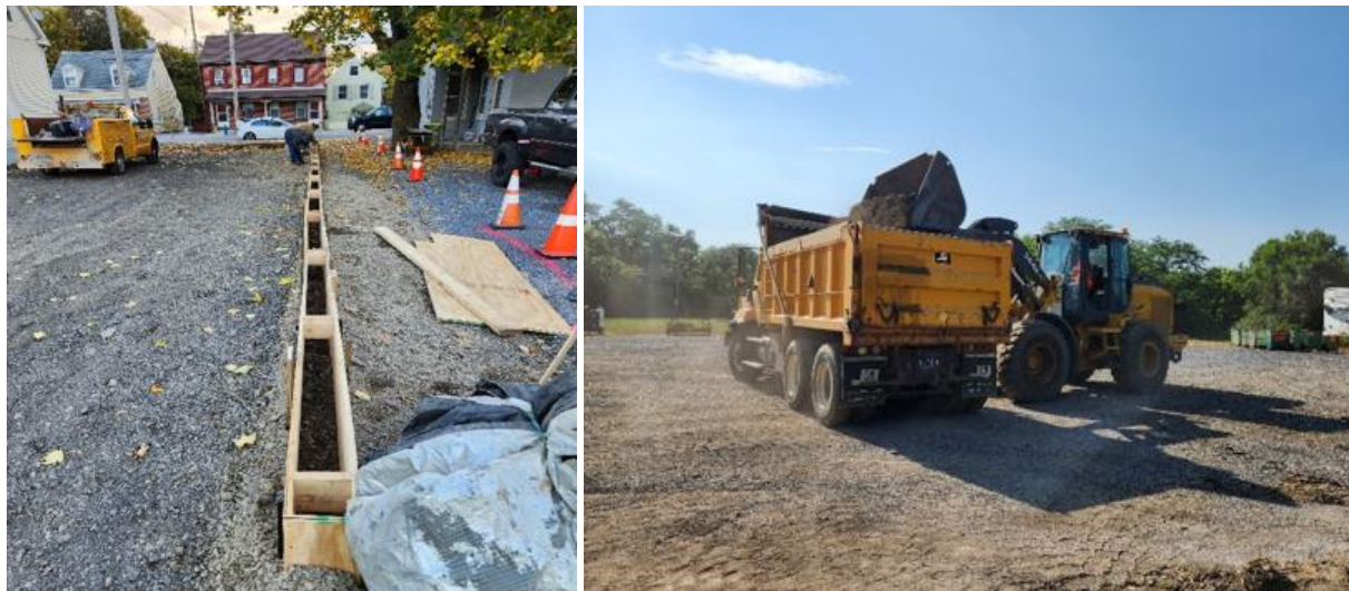
Highway Department Employees Building Curbs and Hauling Materials for Street Paving Projects
