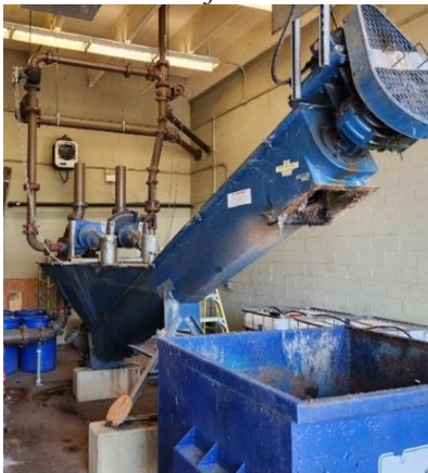
Aging Equipment – Grit Removal
